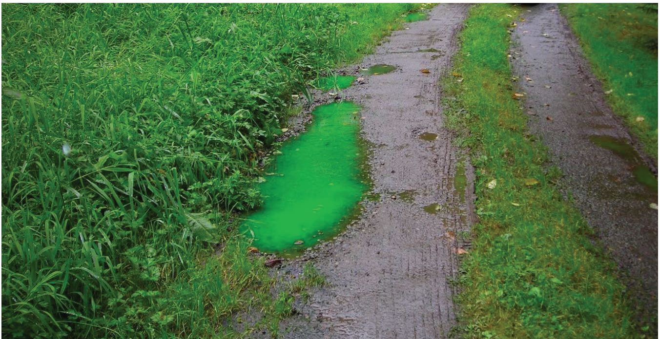
A failure can be confirmed with a fluorescent dye test.
